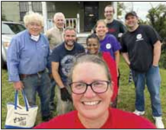
Volunteers from Living Peace Church (Michigan District) removed flood-damaged carpet and other items from this house in Detroit.
