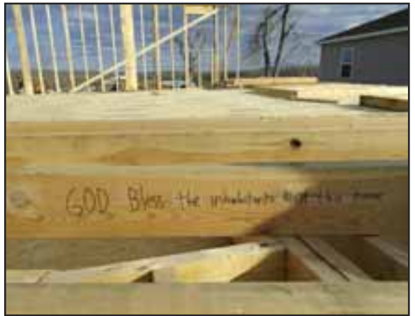
Volunteers pray for future homeowners and often write prayers, Bible verses, and messages of hope on the lumber framing the structure.
